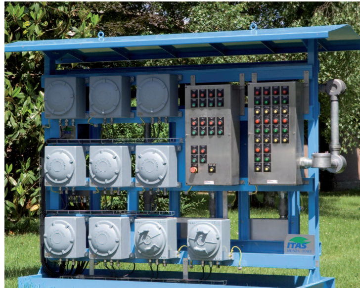
BMS LOCAL PANEL
