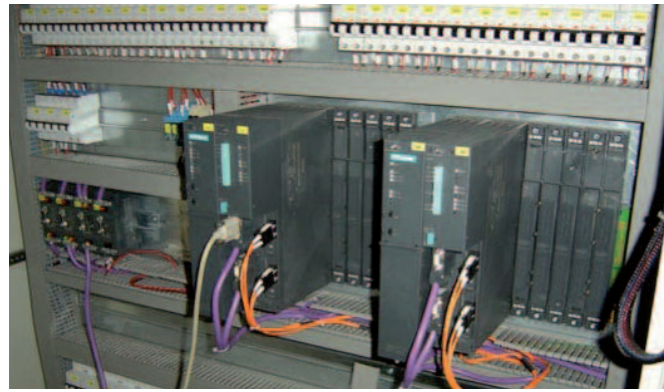
CONTROLLER SIMATIC S7 FAIL SAFE
