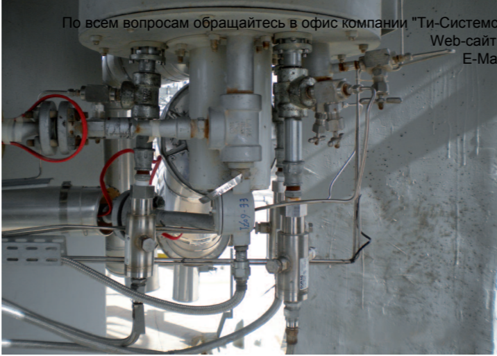
UV+IR SCANNER INSTALLATION ON INCINERATOR BURNER
